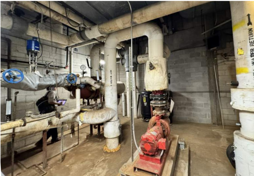
4 Existing mechanical room in natatorium building
