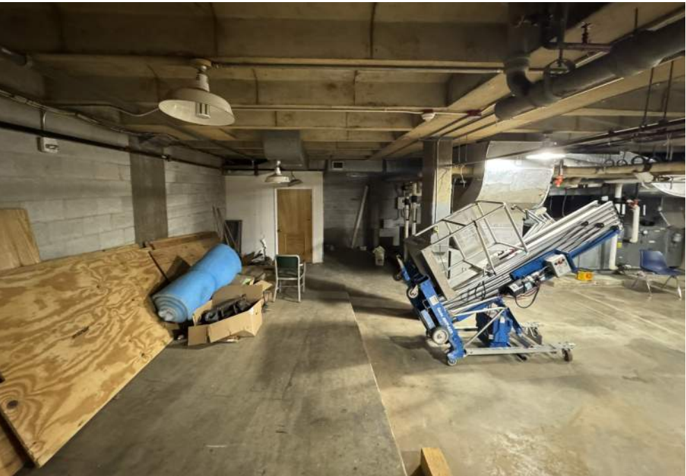
6 Existing mechanical room, to remain
